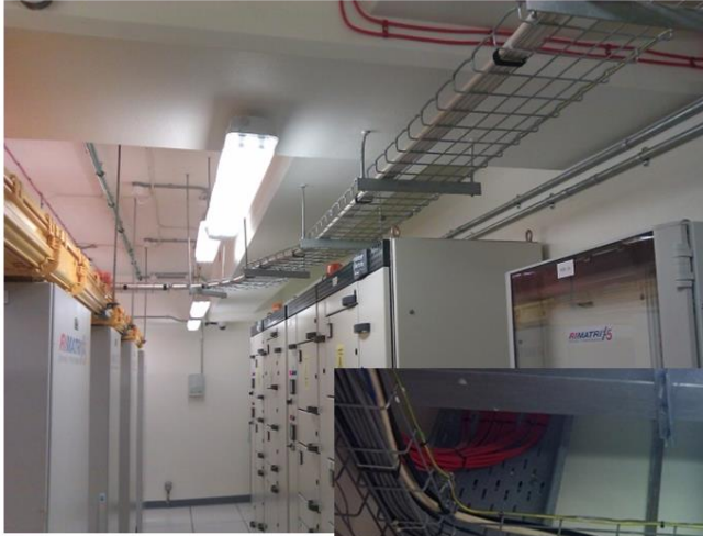
Data Centre connecting the building with 4 fibre cables.
